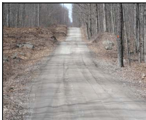
Pine Flats Road - PA Bureau of Forestry
